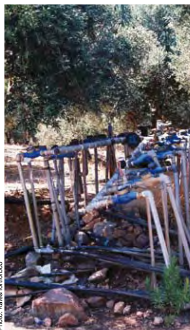
Olive yields are greatly increased through irrigation.
